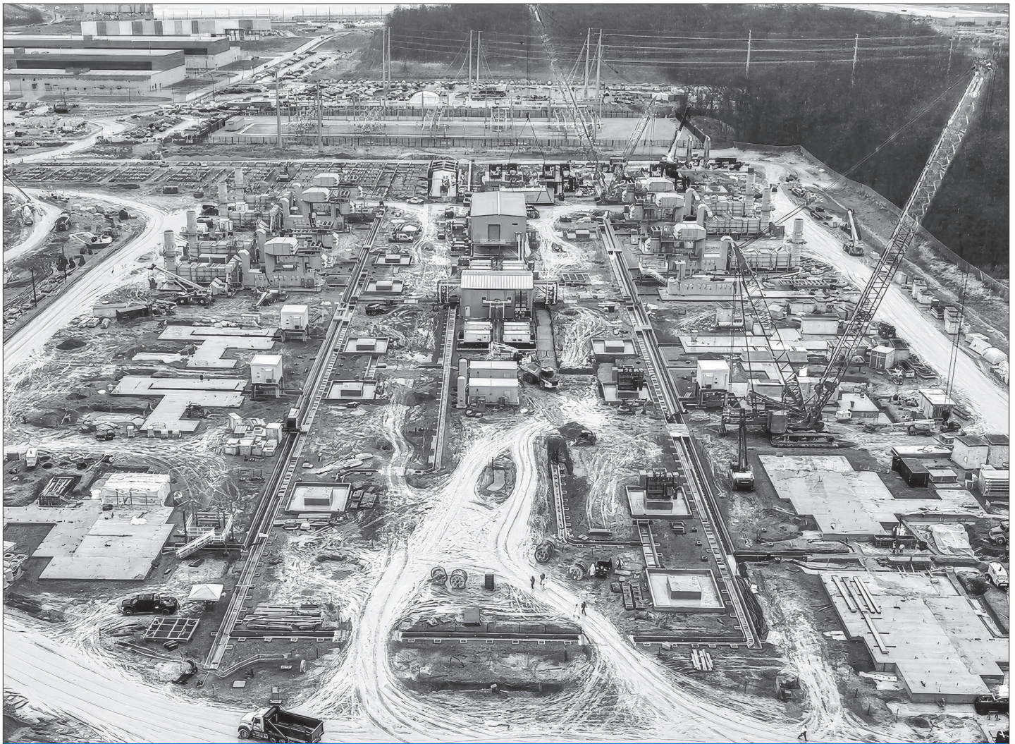
Socrates Power Solution Facility, New Albany, Ohio
